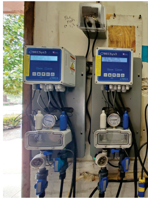
New Pool Chemical Distribution Controls BECSys3 Technology
