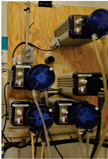
Old Pool Chemical Distribution Controls
